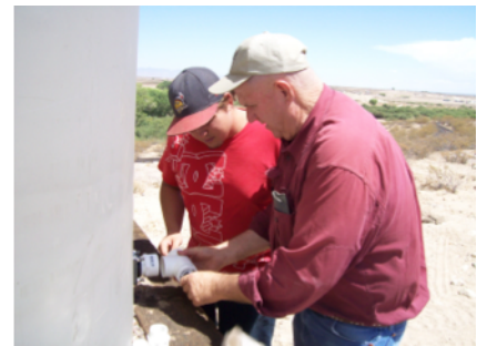
Graham County Extension Director Bill Brandau working with UA extern installing a rainwater harvesting tank.
